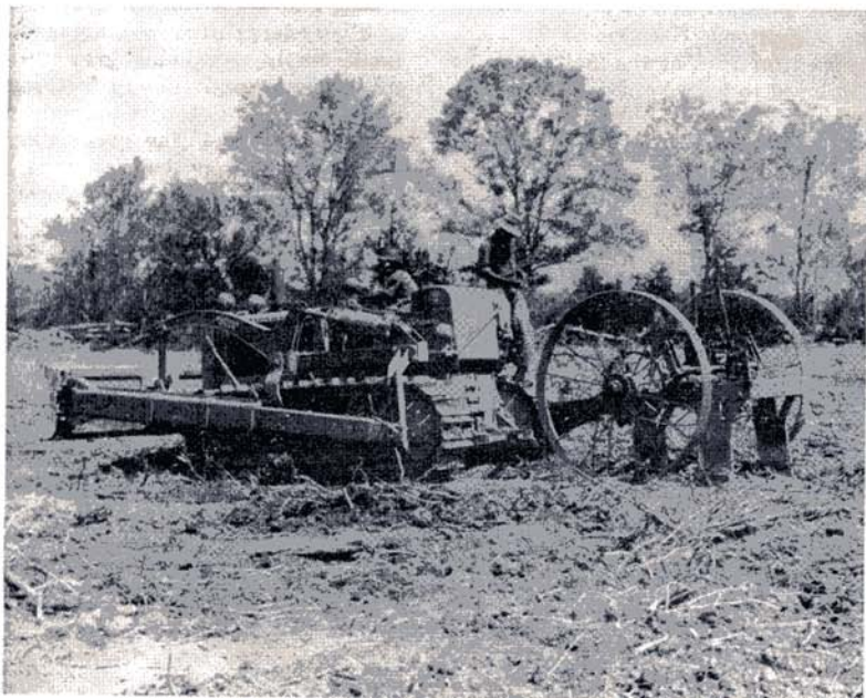
Photo No. 12. International TD 14 equipped with Bucyrus Erie Bull Dozer pulling a root plow.
